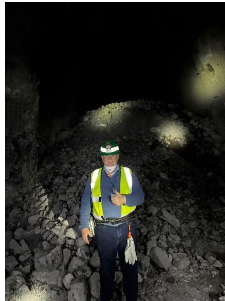
Lift 1 Panel 1 underground development work on Shivee Tolgoi mining license. Source: Entrée Resources Ltd. files January 2025.
